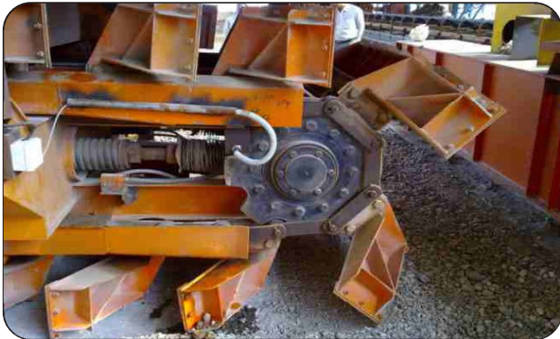
Limestone / Coal Scraper Reclaimer
