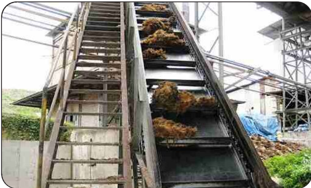
Palm Oil Elevator
