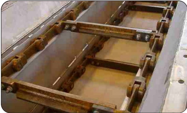
Coal / Ash Feeder
